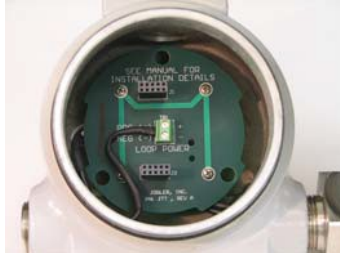
Photograph No. 2 Termination Board
